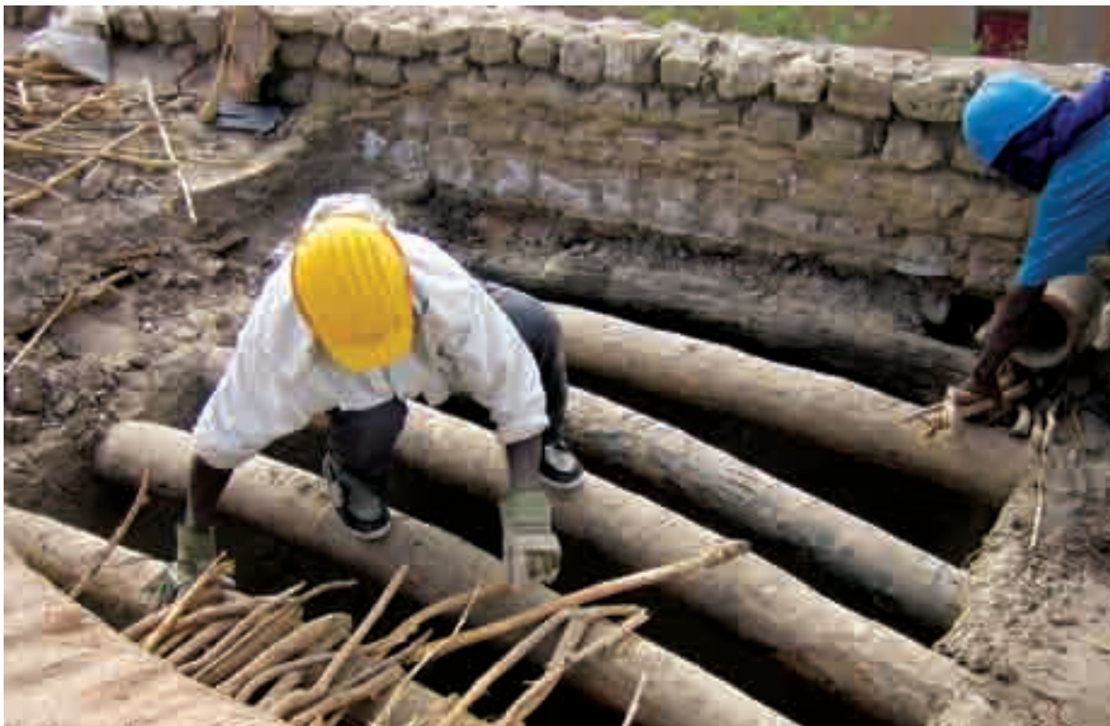
A facade of the mosque and ongoing restoration work. Djingareyber, or the Great Mosque, is Timbuktu's oldest monument and its major landmark. Located at the western corner of the old town, the mosque is almost entirely built in raw earth which is used for mud bricks and rendering.
