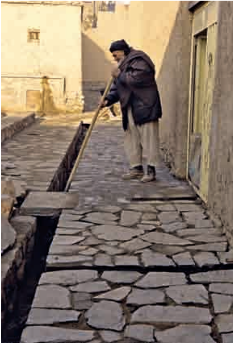
Two images of pavement and drain works (after restoration, top) in the Old City of Kabul near the Babur Gardens.
