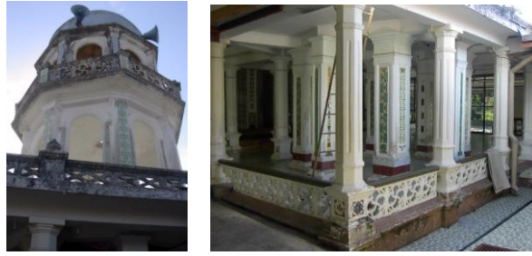
Figure 11: (a) Kampung Rim mosque's tower; (b) Group of column supporting the tower
