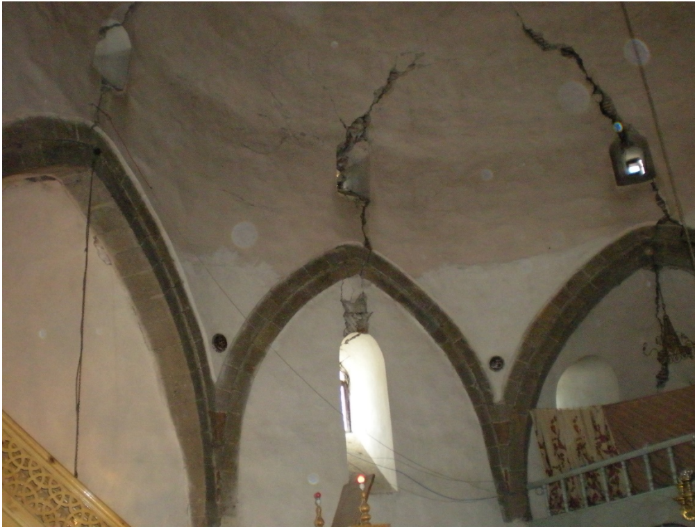
Figure 6. Serious damage in Erzurum Bardız Mosque (Doğangün and Acar, 2009).
