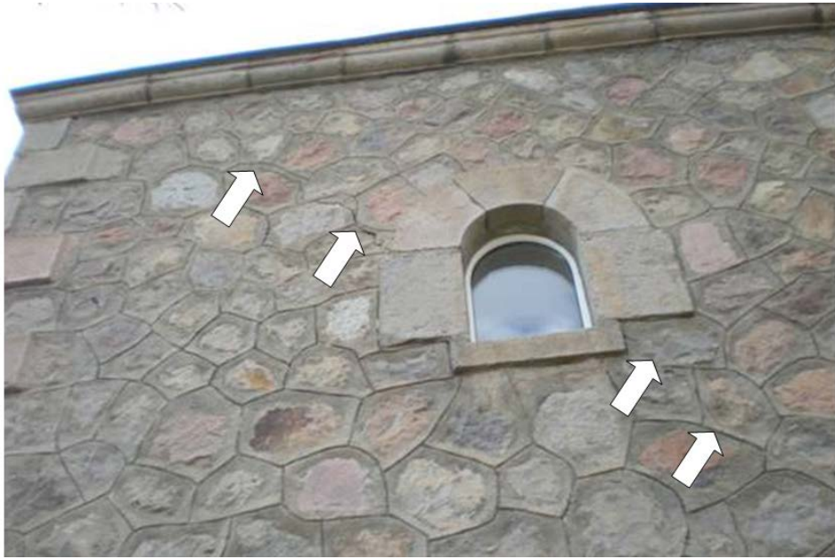
Figure1. Damage on the masonry wall of Kol Mosque in Posof District of Ardahan Province (Doğangün and Angın, 2009)
