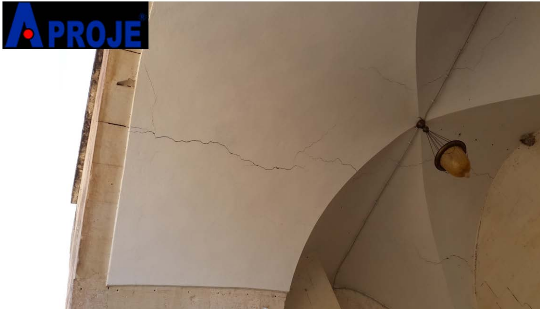
Figure 2. Damage to the Urfa Halfeti Mosque (Doğangün and Livaoglu, 2015).
