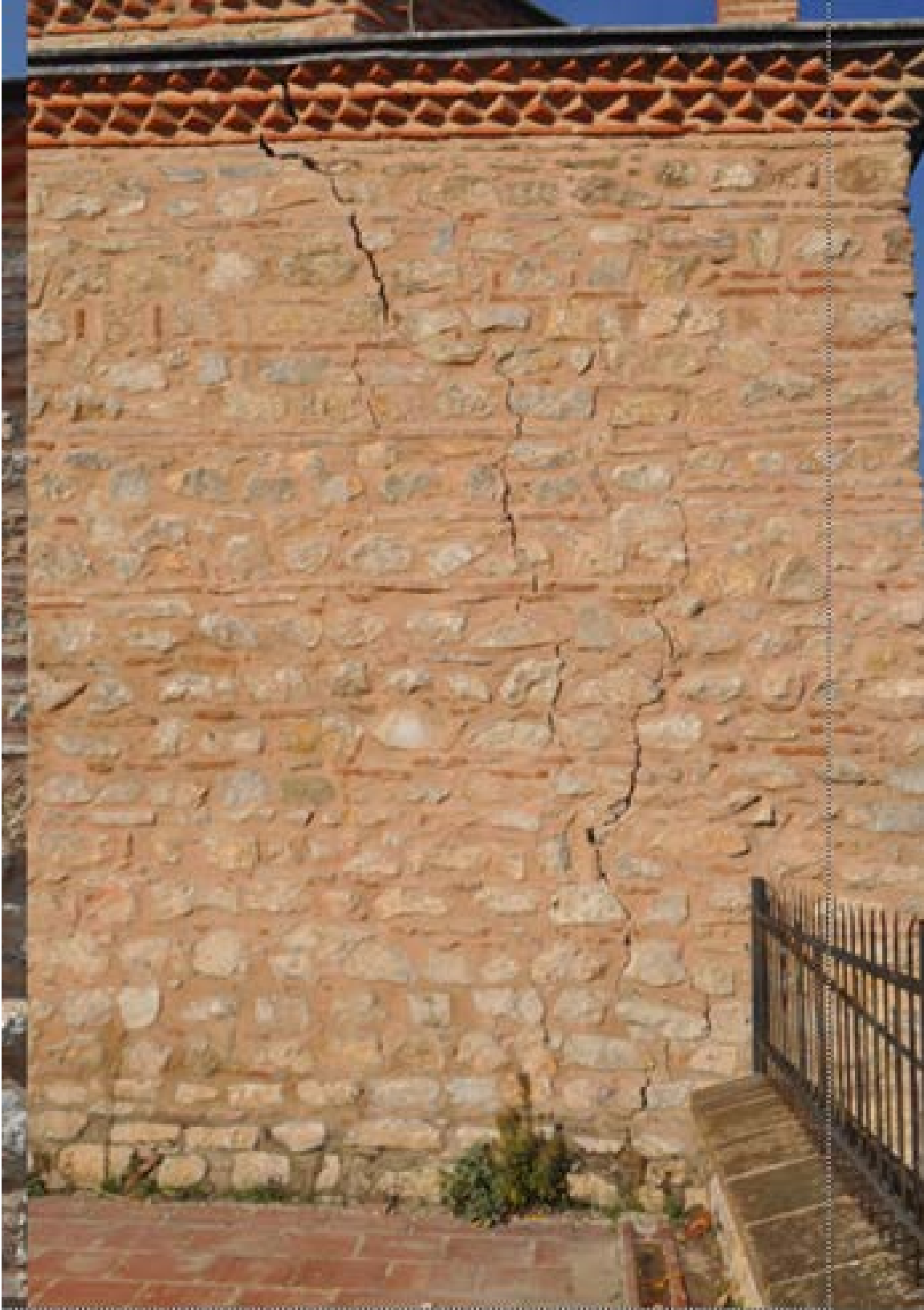
Figure 3. Crack on the wall of Bursa Sinan Pasha Madrasa (Livaoğlu and Doğangün, 2014)
