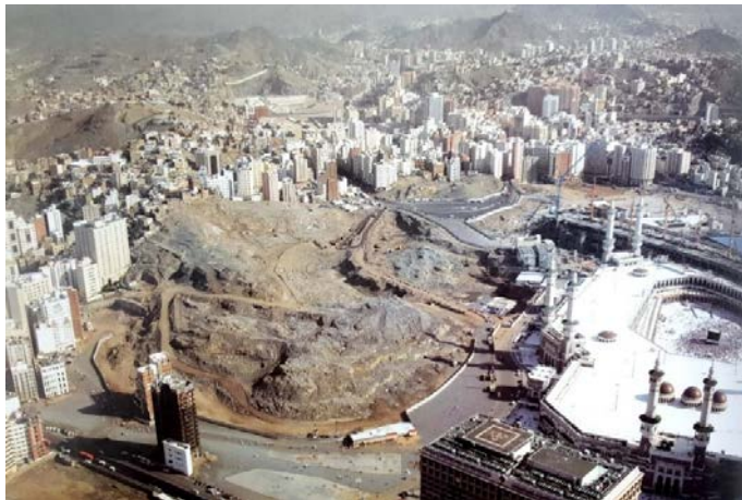
Figure 9: The demolishing area in the northern side to expand the Holy Mosque. (Source: Mirza, 2016, p. 301.)
