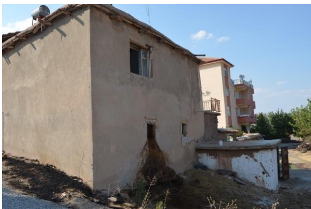
Figure 2. A traditional building that has partially lost its originality with a concrete plaster in Bahri and a reinforced concrete structure adjacent to this structure (30.08.2017)
