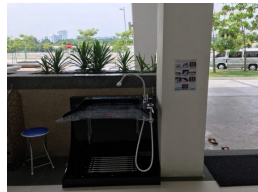
Figure 8: Ablution installation (Source: author)
