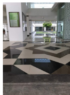
Figure 9: slippery floor tiles at the prayer hall (Source: author)
