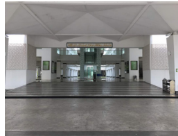
Figure 5: main entrance with slippery tiles (Source: author)
