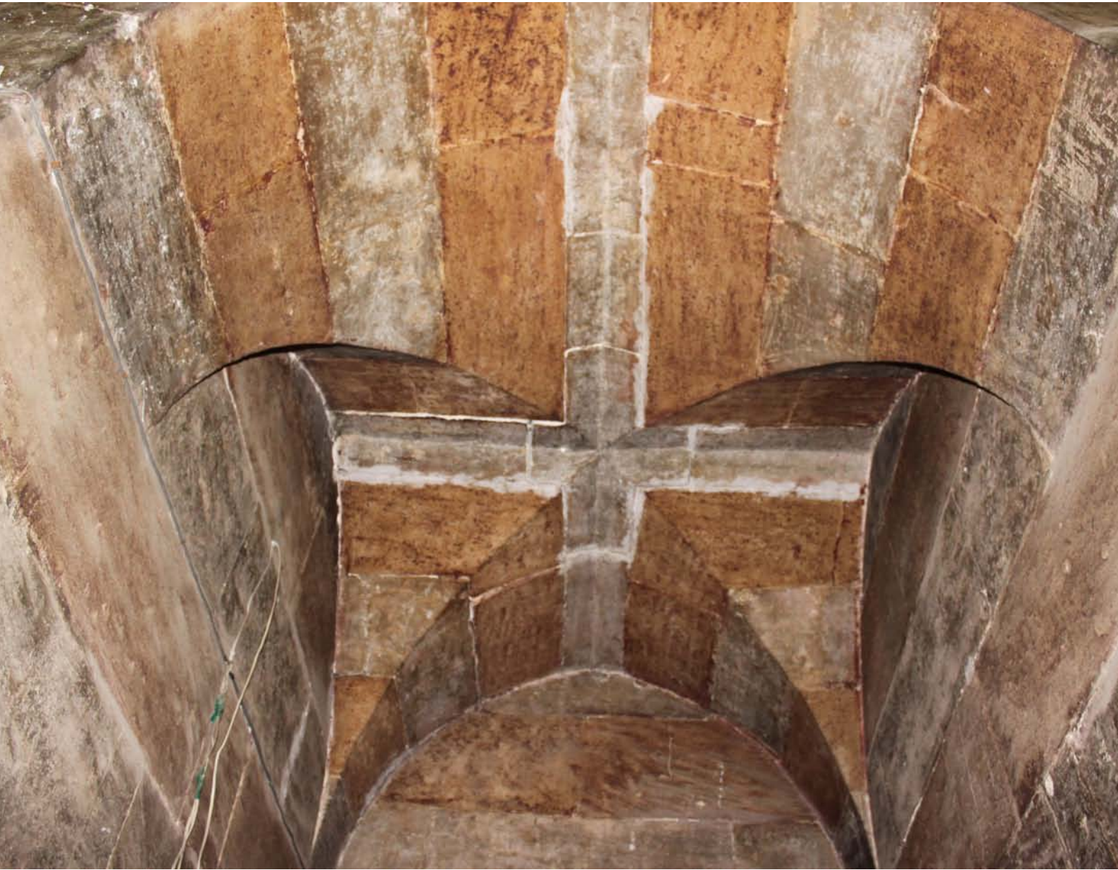
Fig. 4.54: Groin vault with the cruciform on the ceiling of the stairs leading to the ablution corridor
